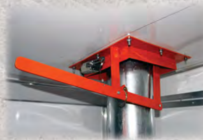
Exhaust Vent With Burner Safety Switch
